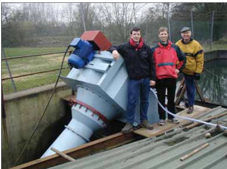
(h) A 15 kW siphon turbine demonstration in the UK.
