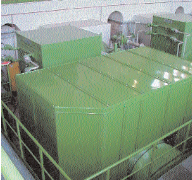
Noise reduction systems installed on a turbine STUDIO FROSIO
